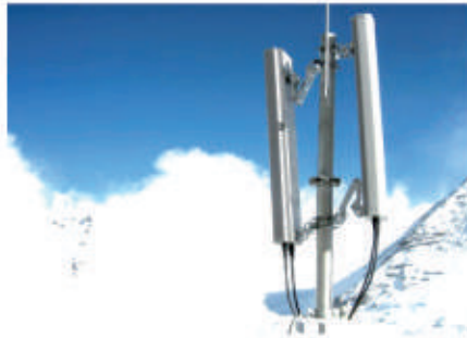
基站信号中转站 Base station signal relay station
